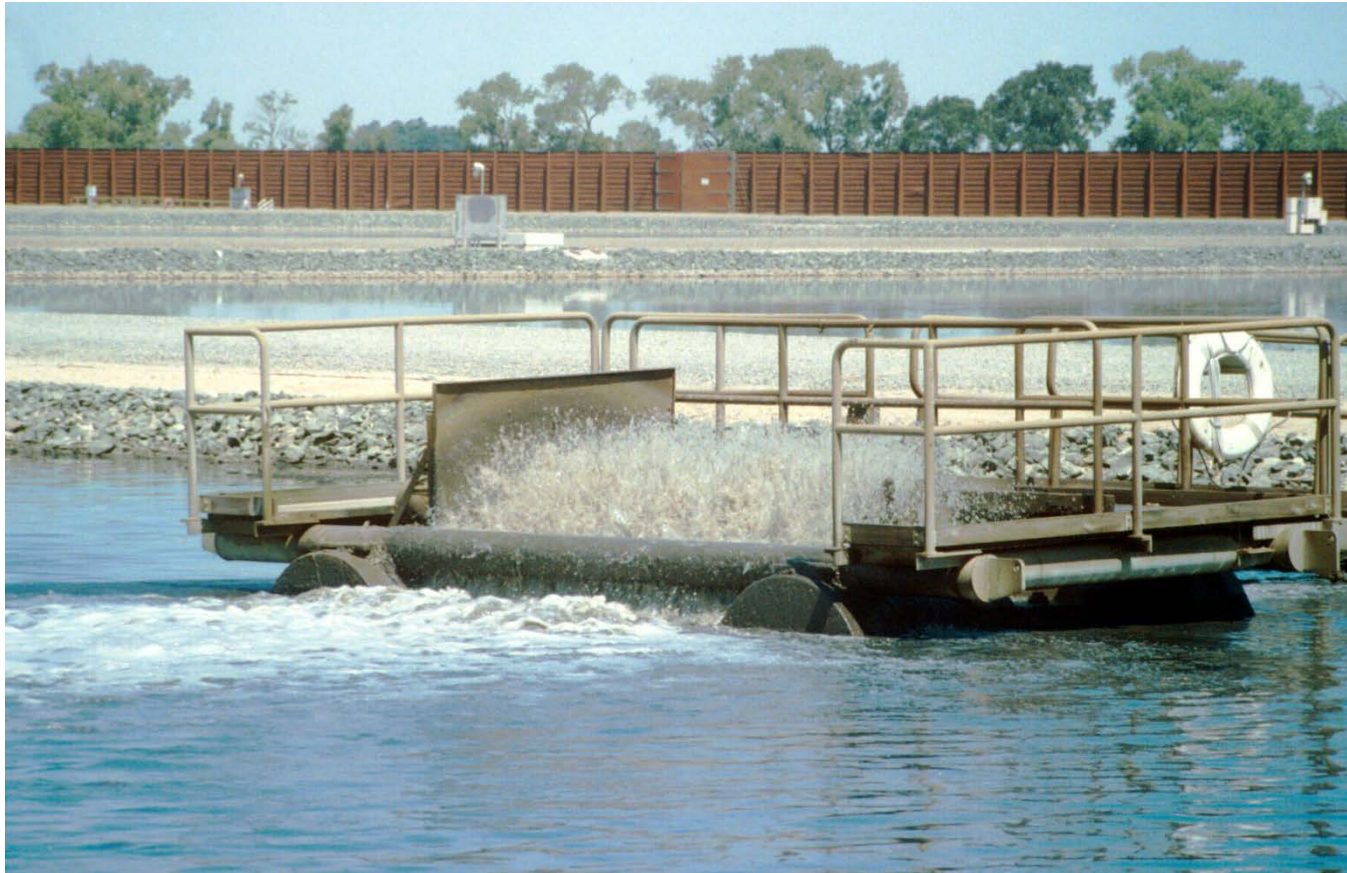
Floating brush aerator provides mixing in a large lagoon
