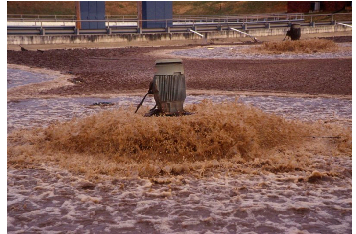
In an activated sludge tank
