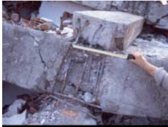
Fig. 10 Beam-column joint damage – bar slip
