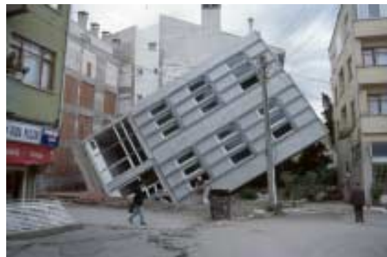
Fig. 18 Liquefaction induced bearing failure in Adapazari
