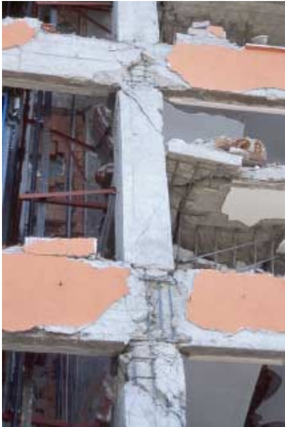
Fig. 9 Beam-column details and damage
