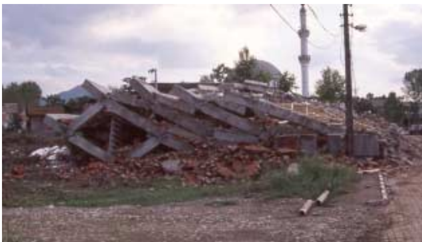
(a) Complete collapse of building west of Gölcük
