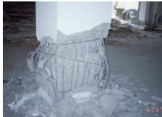
Fig. 11 Column compression failure
