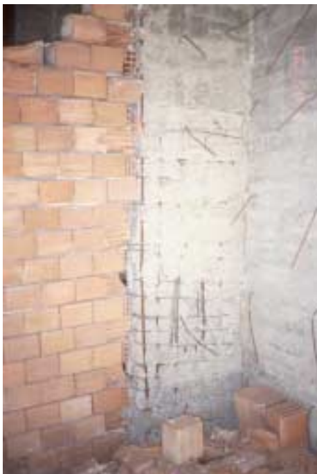
Fig. 16 Poor concrete placement In shear wall (Yalova)
