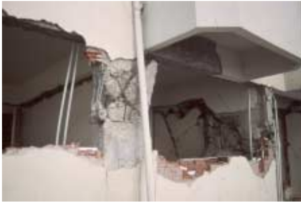
(a) Column shear failure (wall in background)
