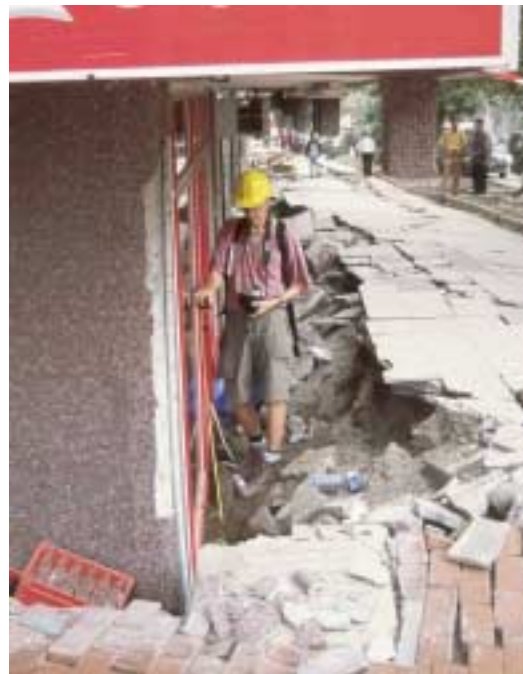
Fig. 17 Bearing/settlement failure in Adapazari
