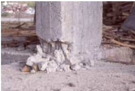
Fig. 15 Bent column bar at foundation
