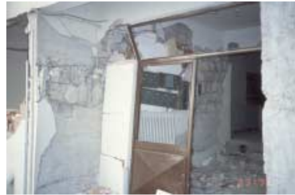
(b) Shear failure in coupled wall
